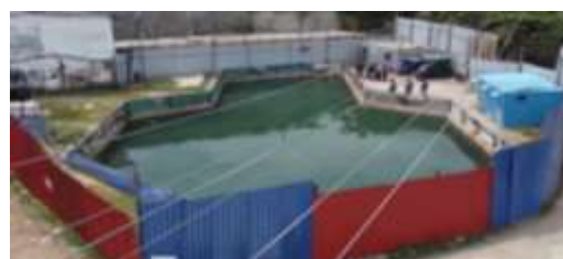
Thalakotuwa Garden Pumping Station
