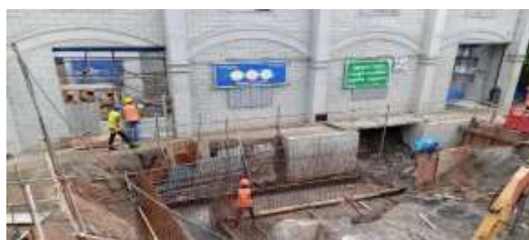
Thimbirigasyaya Pumping Station
