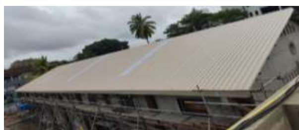
Borella Pumping Station
